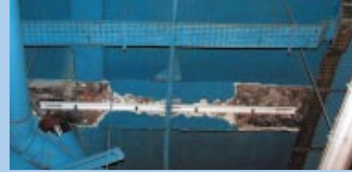
Optic cable on steel beam dating to 1853
