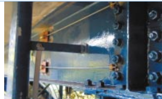
Installed optical Strands on the main bridge support.
