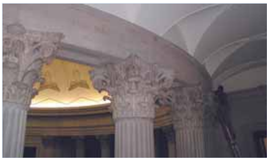
The way taken by the optical link cable on the rotunda is totally invisible.
