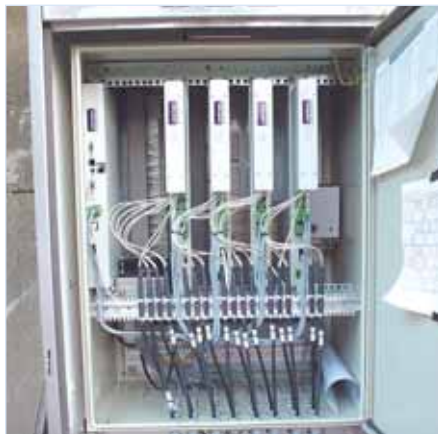
Monitoring station connected to the OSMOS Internet databank server.
