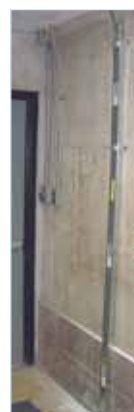
One of the 4 optical strands of the global tiltmeter.
