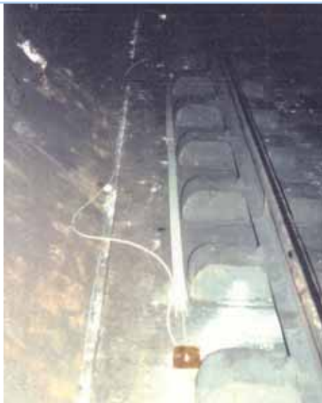
The length of an optical strand should be greater than the Z of the tunnel in order to determine its behaviour as a beam on between two elastic bearing points.
