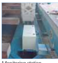
Monitoring station connected to the OSMOS database server.
