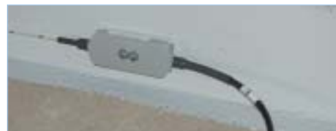
Detail of an Optical Strand at the level of connection to the fiber optic network
