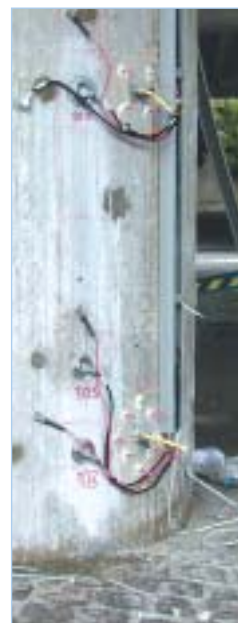
Hygrometers and corrosion sensors
