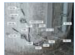
Hygrometers and corrosion sensors (detail)
