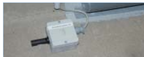
Flood detector in plumb with an Optical strand
