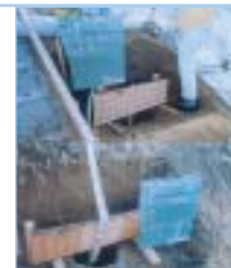
Panels arranged in staggered rows
