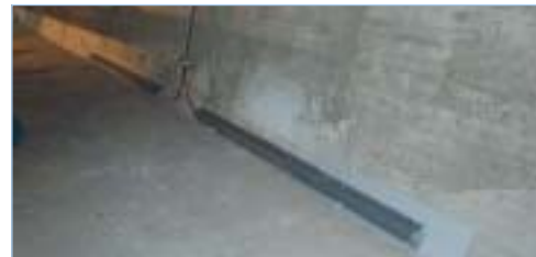
Dual 2-meter Optical Strands inside bridge deck
