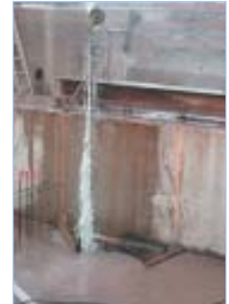
Sectionning of a crossbrace
