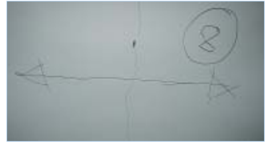
Marking of the cracked zones prior to installation
