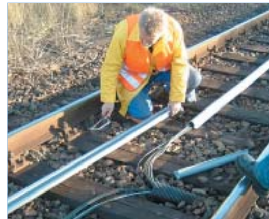
The optical link cables lead to the monitoring station
