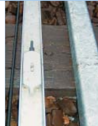
Optical strand on steel mounting plate, prior to installation of protective housing
