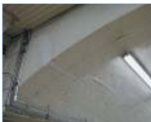
Optical strand under one of the rail lines, prior to installation of protective housing
