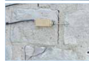
Close-up view of an optical extensometer on vertical cracks
