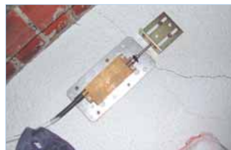
Extensometers and optical feelers are installed inside and outside the edifice before the start of the works
