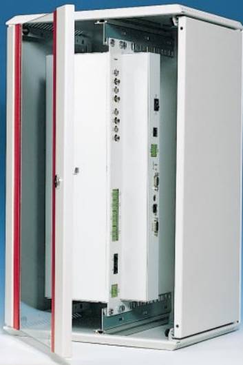
Monitoring station in a cabinet.
