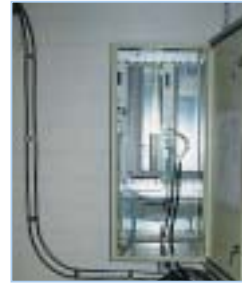
Station de monitoring
