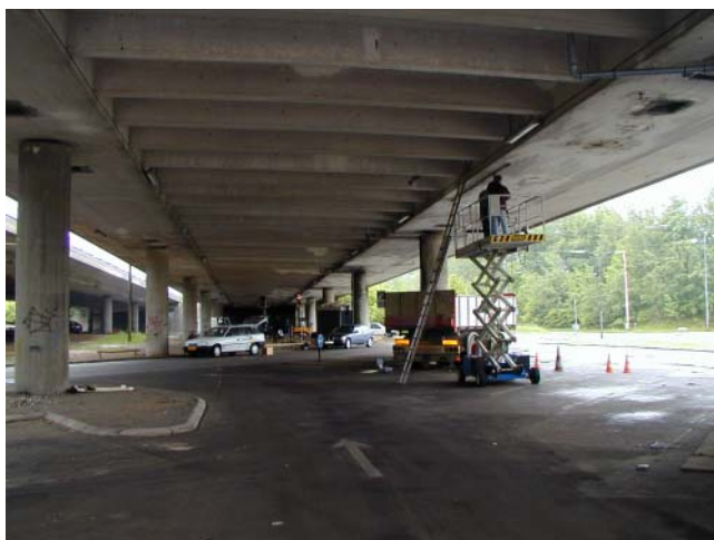
Fig. 11: Mounting a 5-m long OSMOS fiber-optic deformation sensor under a girder, mid-span.
