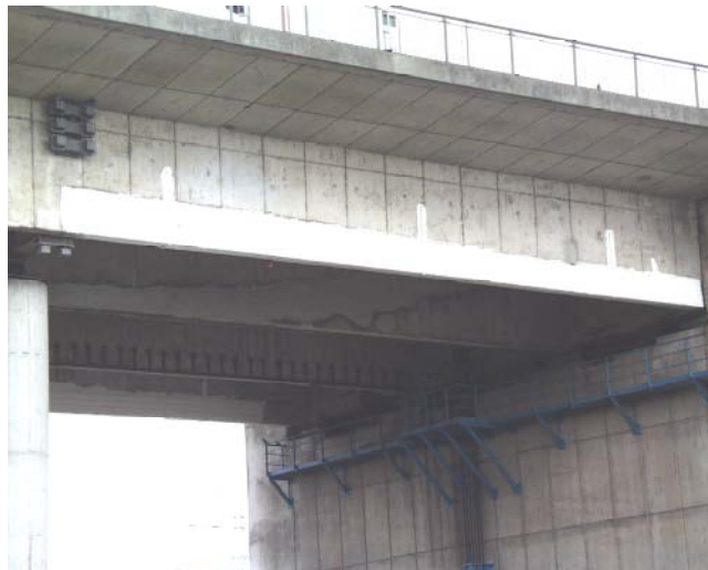
Fig. 13: Position of four 5-m long OSMOS fiber-optic deformation sensors on the side of the girder in the weak part of the Herrenbrücke, Lübeck.
