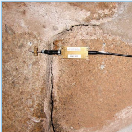
Extensometer as a fissure monitor.
