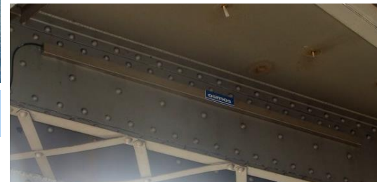
Optical Strand on the upstream anchoring beam, with cover protection
