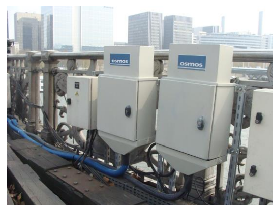
Monitoring Station installed on the Viaduct, near the Austerlitz Station
