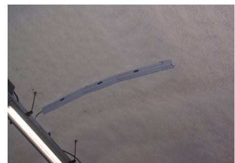
Optical Strand's installation on the tunnel underface vault with it PVC protection
