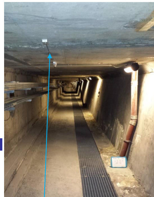
LIRIS Optical Strand on the slab underface
