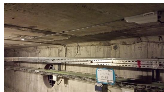
LIRIS Optical Strand on the slab underface
