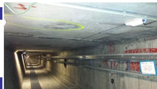
LIRIS Optical Strand on the slab underface
